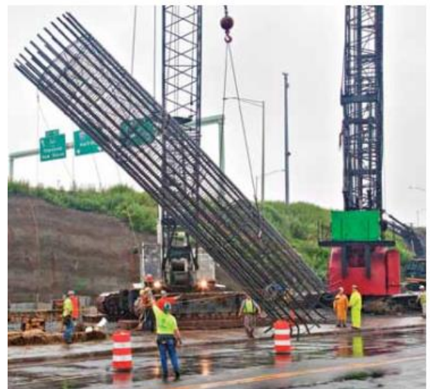
Fig. 7: A well-braced drilled shaft cage is picked with minimal distortion (photo courtesy of Dimension Fabricators, Inc.)
