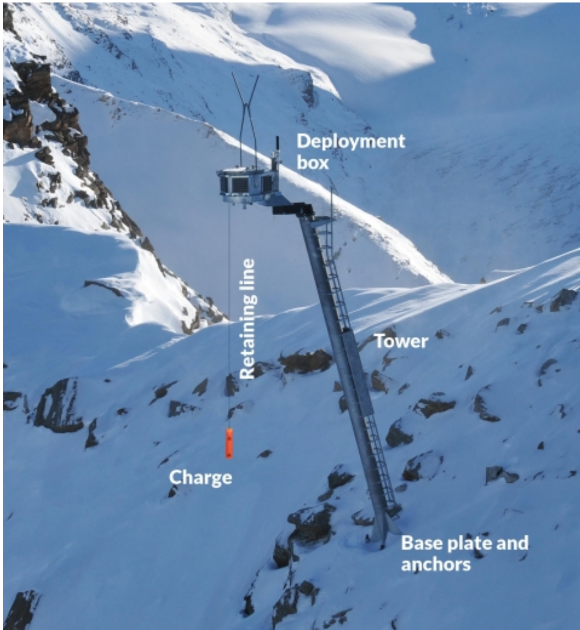
Figure 2: The avalanche tower can be remotely activated to lower a charge to a specified height above the snow. The deployment box can be stocked with multiple charges, obviating the need for restocking during the avalanche season.
