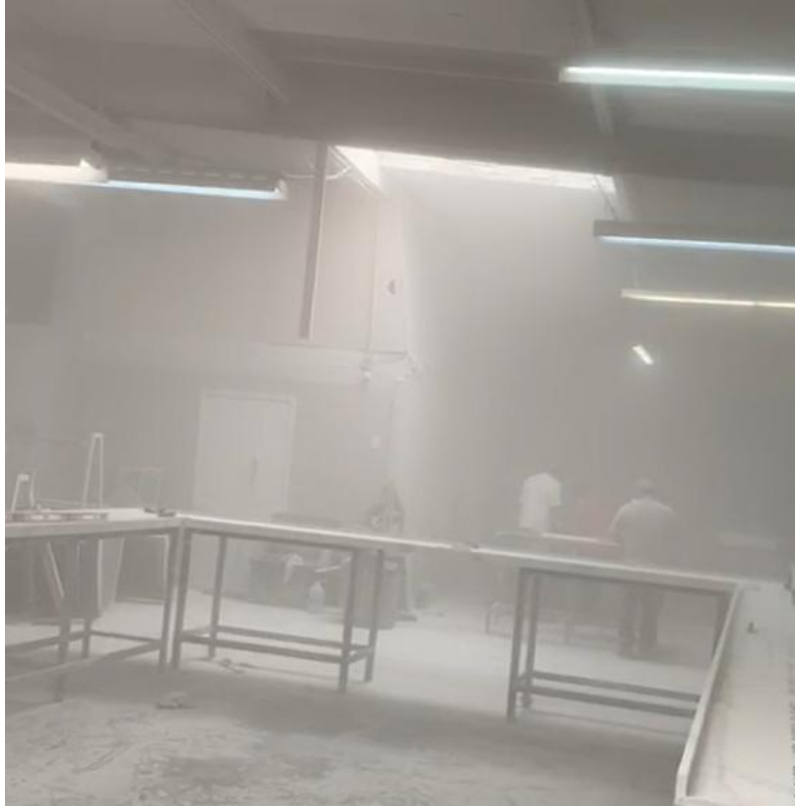
Plate 3. A general view of the shop interior. Airborne dust obscures visibility across the width of the building. Exposure at this density is not confined to the operator performing the task. Every person present is breathing it, including those performing no cutting at all.
