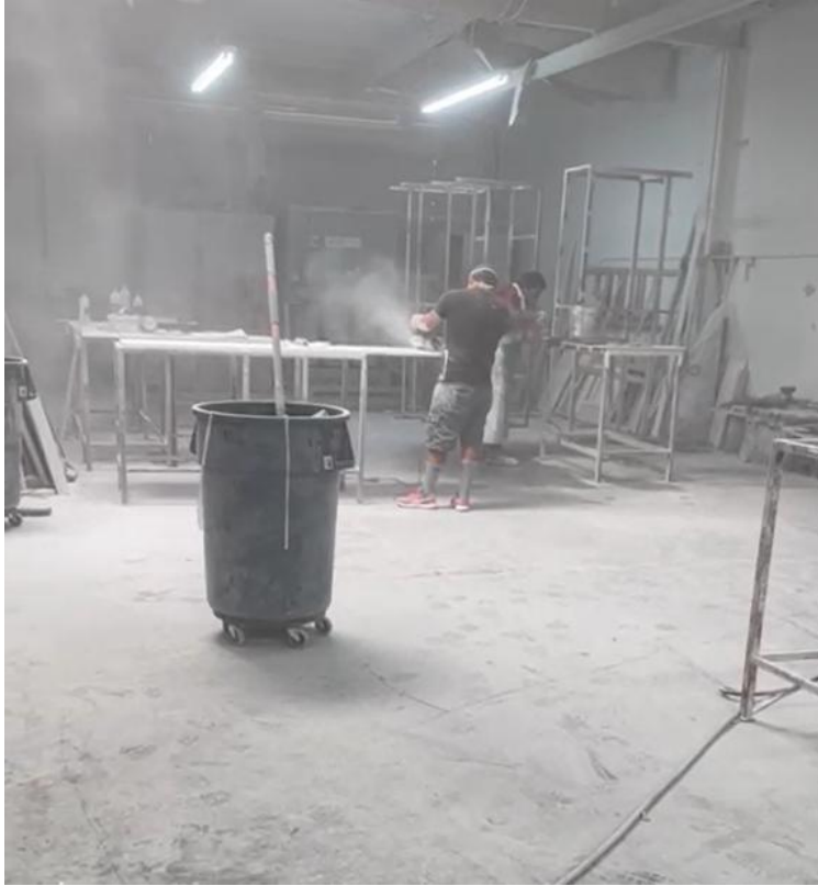
Plate 4. A second general view. Dust is generated at a work table with no water suppression and no capture at source, and has settled across the floor and the surrounding surfaces, where ordinary movement will return it to the air.
