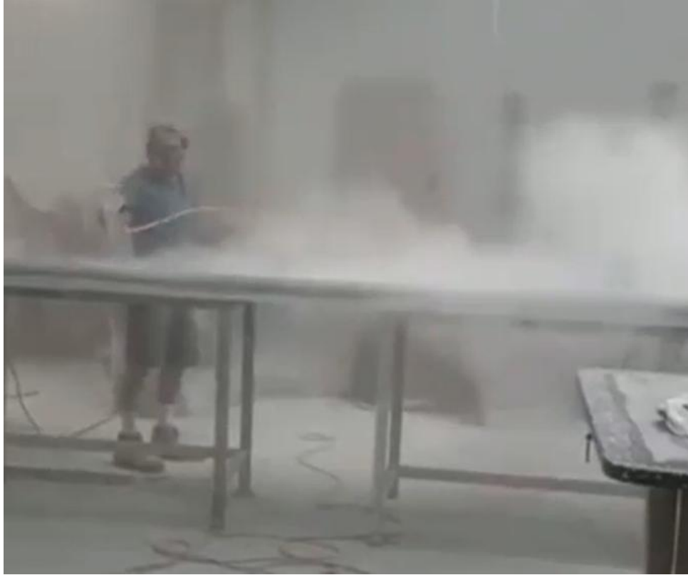
Plate 2. Dust is being cleared from a slab by blowing rather than by wet methods or a HEPA vacuum. Section 5204(f)(2)(D) prohibits the use of compressed air on materials that may contain crystalline silica, and prohibits dry clean-up of such materials.
