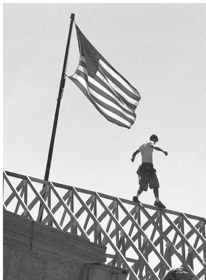
DLSE and Cal/OSHA investigators conduct enforcement sweeps in residential construction projects to combat widespread labor law violations. This residential construction worker should be wearing fall protection to prevent a potentially fatal accident.
