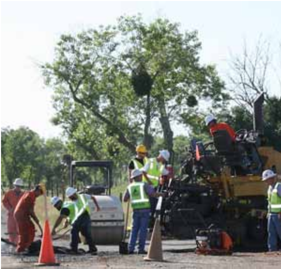
Local 3 apprentices pave the entrance to the new training site in April.
