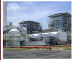
Subcritical Utility Boilers
