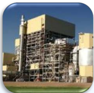
Utility Steam Generation
