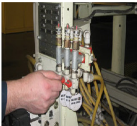
Bleeding air pressure by opening a valve
